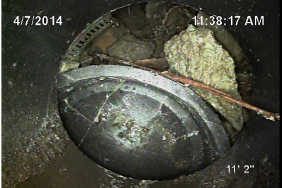
4/7/2014 11:38:17 AM Sewer line not connected at guest house
