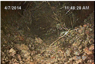
4/7/2014 11:48:28 AM Root intrusion and possible collapsed pipe
