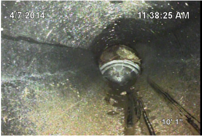
4/7/2014 11:38:25 AM Sewer line not connected at guest house
