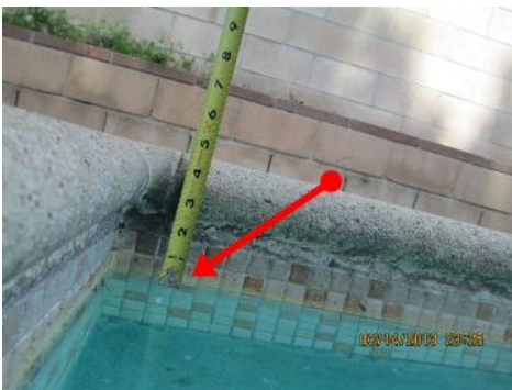
pool out of level south side of pool
