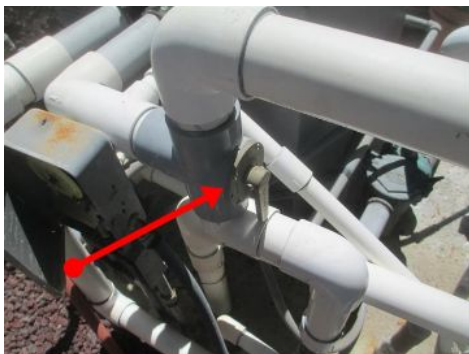
valve is leaking
