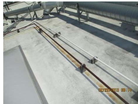
rusted fuel piping observed
