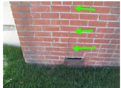
vertical cracking in brick
