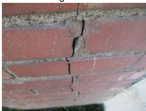
vertical cracking noted
