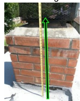
chimney is too short
