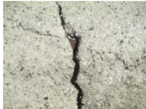
cracks noted in cap
