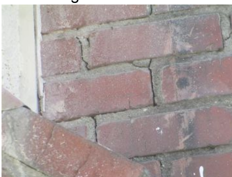
vertical cracking noted
