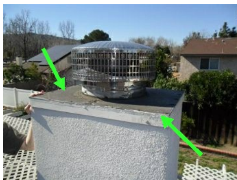
chase cover is field modified in substandard manner
