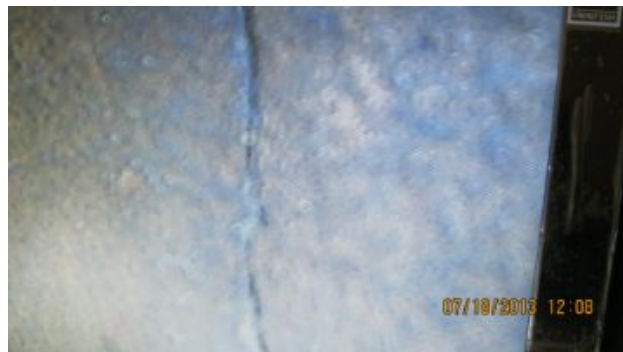
cracks in flue
