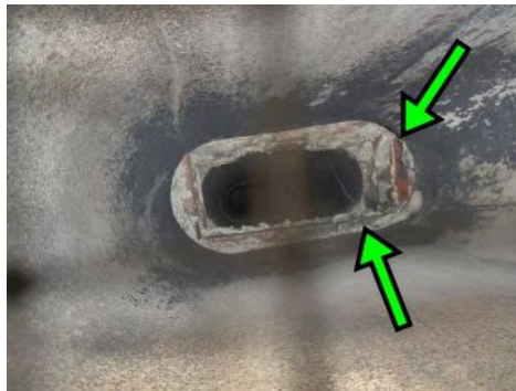
missing flue liner
