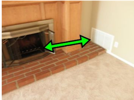
fireplace clearance to return air vent substandard
