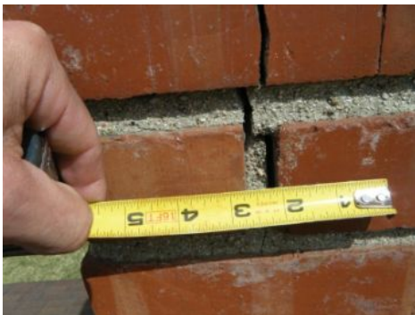
large cracks noted
