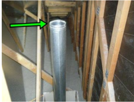
fireplace flue does not penetrate roof
