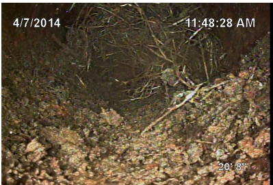
4/7/2014 11:48:28 AM Root intrusion and possible collapsed pipe
