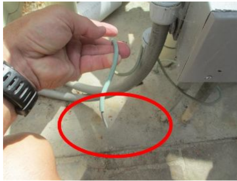
disconnected pool equipotential bonding conductor
