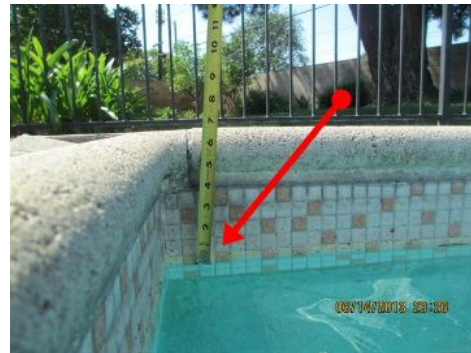
pool out of level north side of pool
