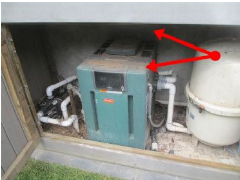
heater clearance to wood is substandard
