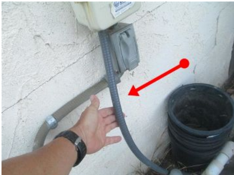
conduit is not secured in accordance to building standard
