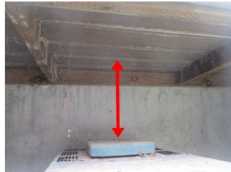
heater clearance to wood is substandard
