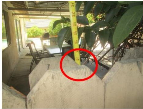
pool barrier is short
