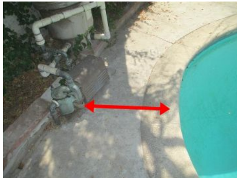
pool equipment is too close to water
