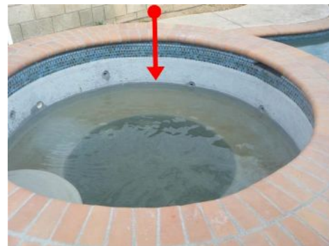
bad "check valve" causing the spa to drain out
