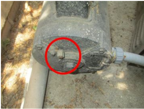
no bond observed at the pool motor
