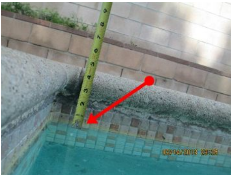
pool out of level south side of pool
