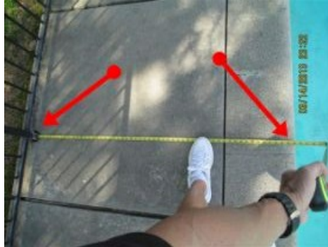
wrought iron fence too close to pool water
