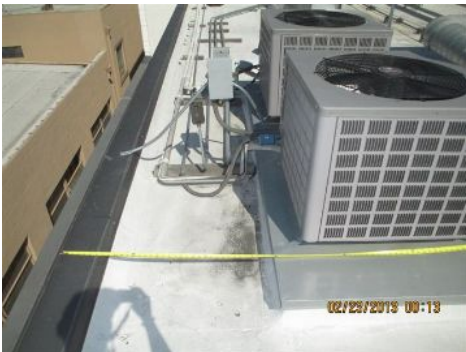
1013.5 Mechanical equipment. Guards shall be provided...
