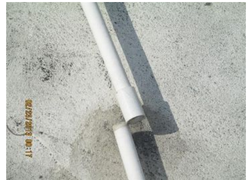
disconnected condensate drain piping
