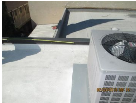
1013.5 Mechanical equipment. Guards shall be provided...
