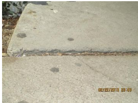
side walk has raised surface
