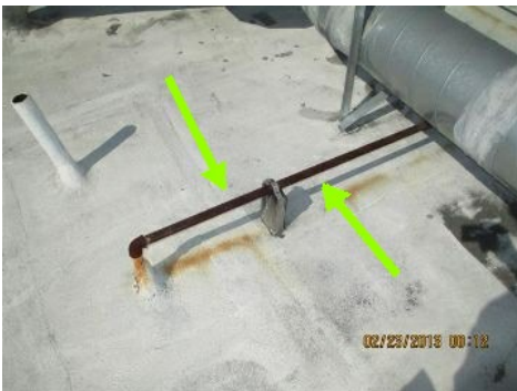
fuel piping is rusted suggested to be painted
